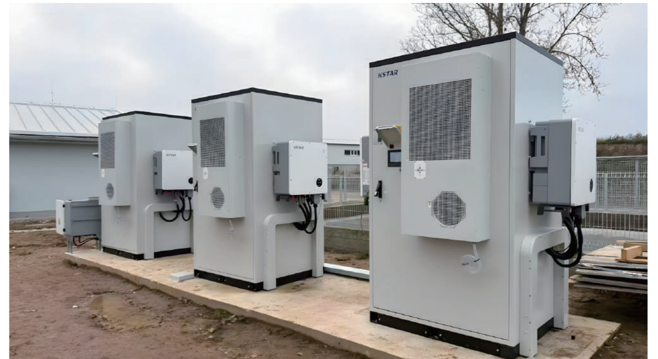
05 C&I ESS Project in Czech Republic
