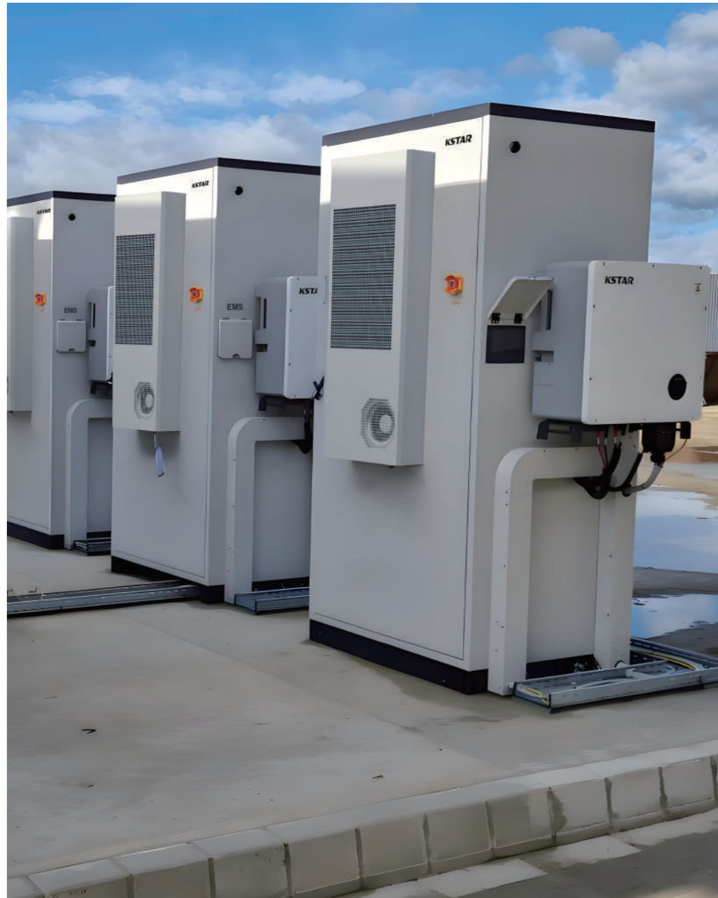
07 C&I ESS Project in Hungary
