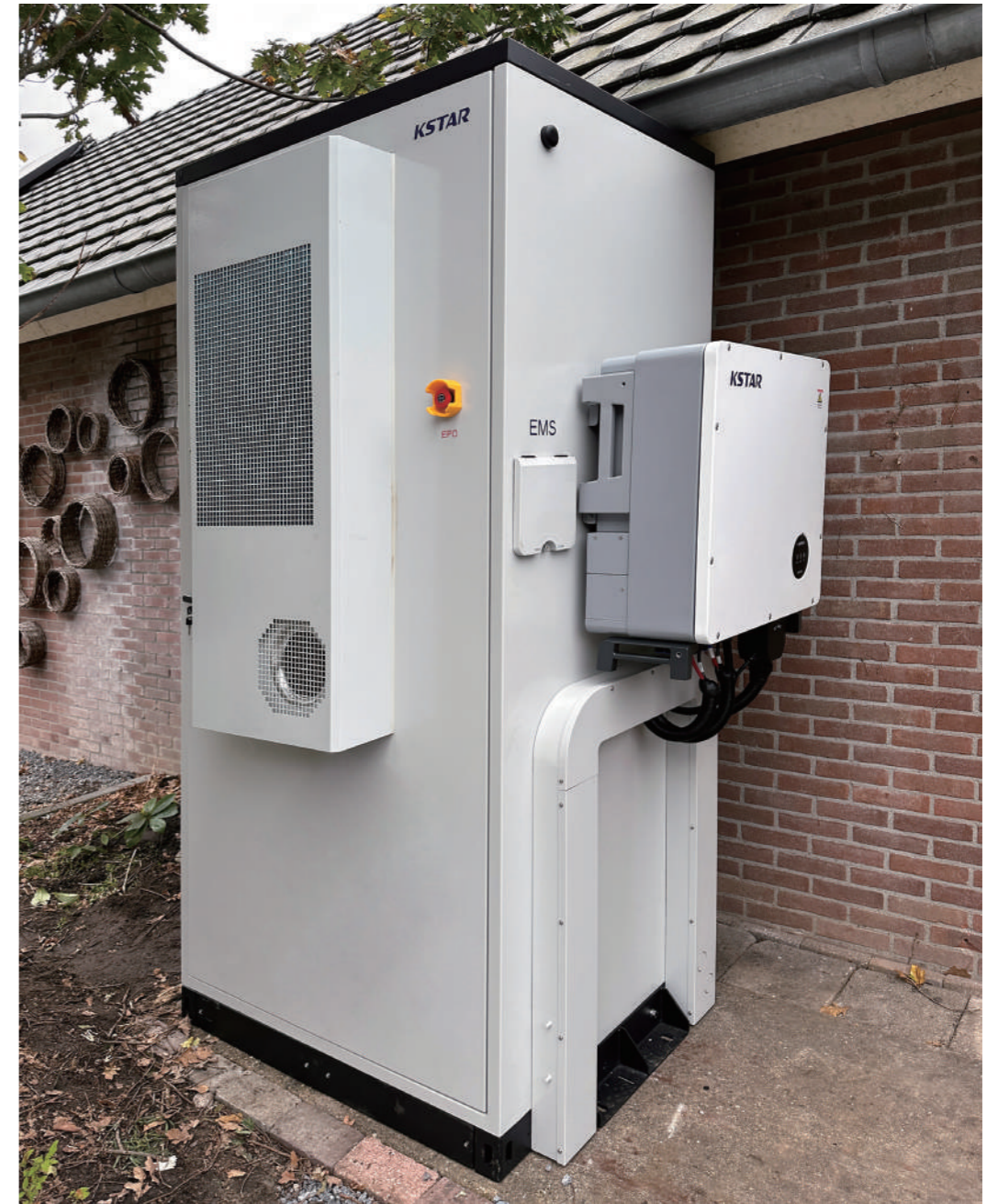
08 C&I ESS Project in the Netherlands
