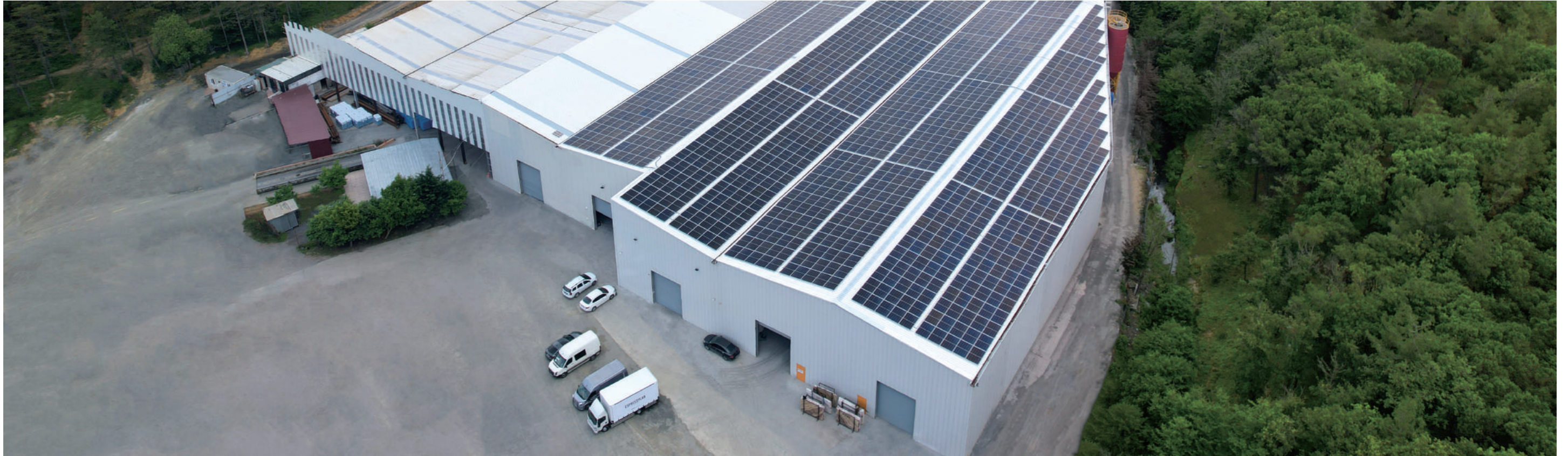
09 Energy Cost Reduction for Mineral Water Factory Turkey, 900kW KSG-120CL-M0
