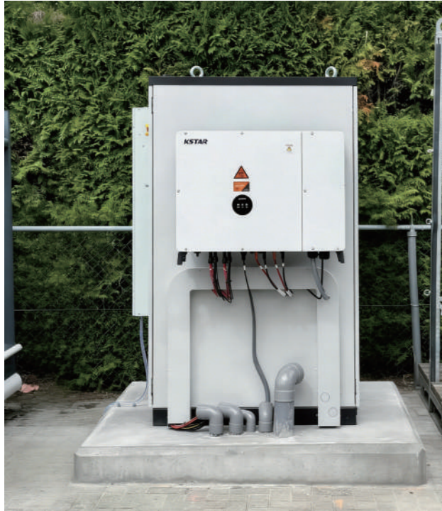
01 C&I ESS Project in the Netherlands
