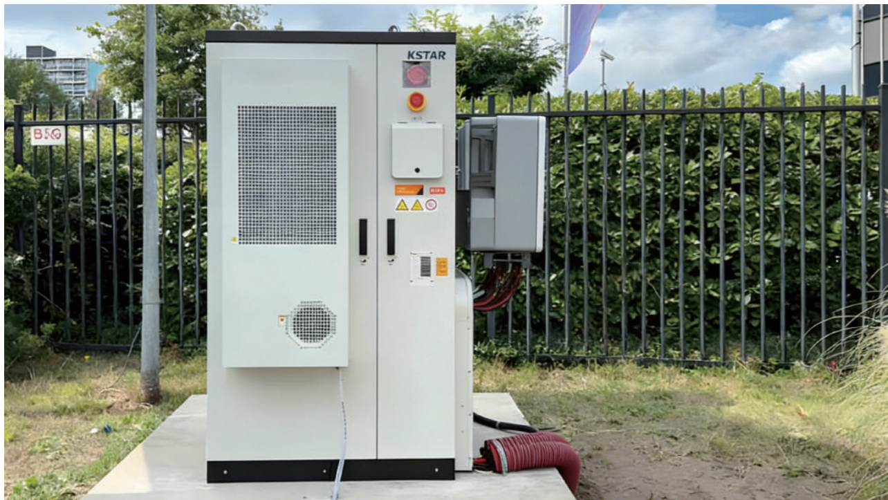
04 C&I ESS Project in the Netherlands
